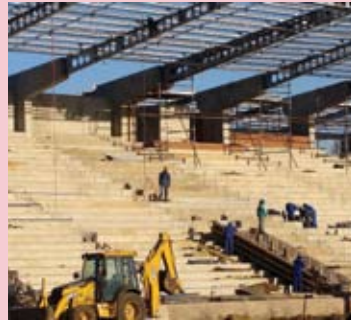
A water repellent produced by a.b.e. Construction Chemicals was used to seal the concrete surfaces of a new pavilion at the Harry Gwala Stadium in Pietermaritzburg.
