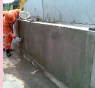
a.b.e. Construction Chemicals General Construction products, durarep FR and durarep FC, are being used for concrete repairwork on Gautrain viaduct cable trenches.
