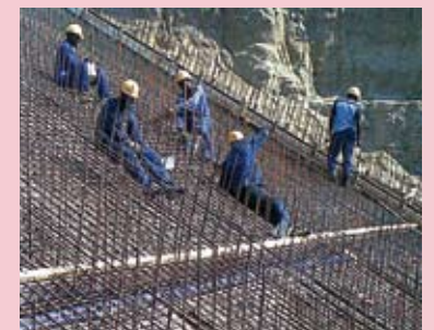
a.b.e.'s durajoint PVC waterstop was used to seal the joints during the upgrading of the Gaborone wastewater treatment project.
