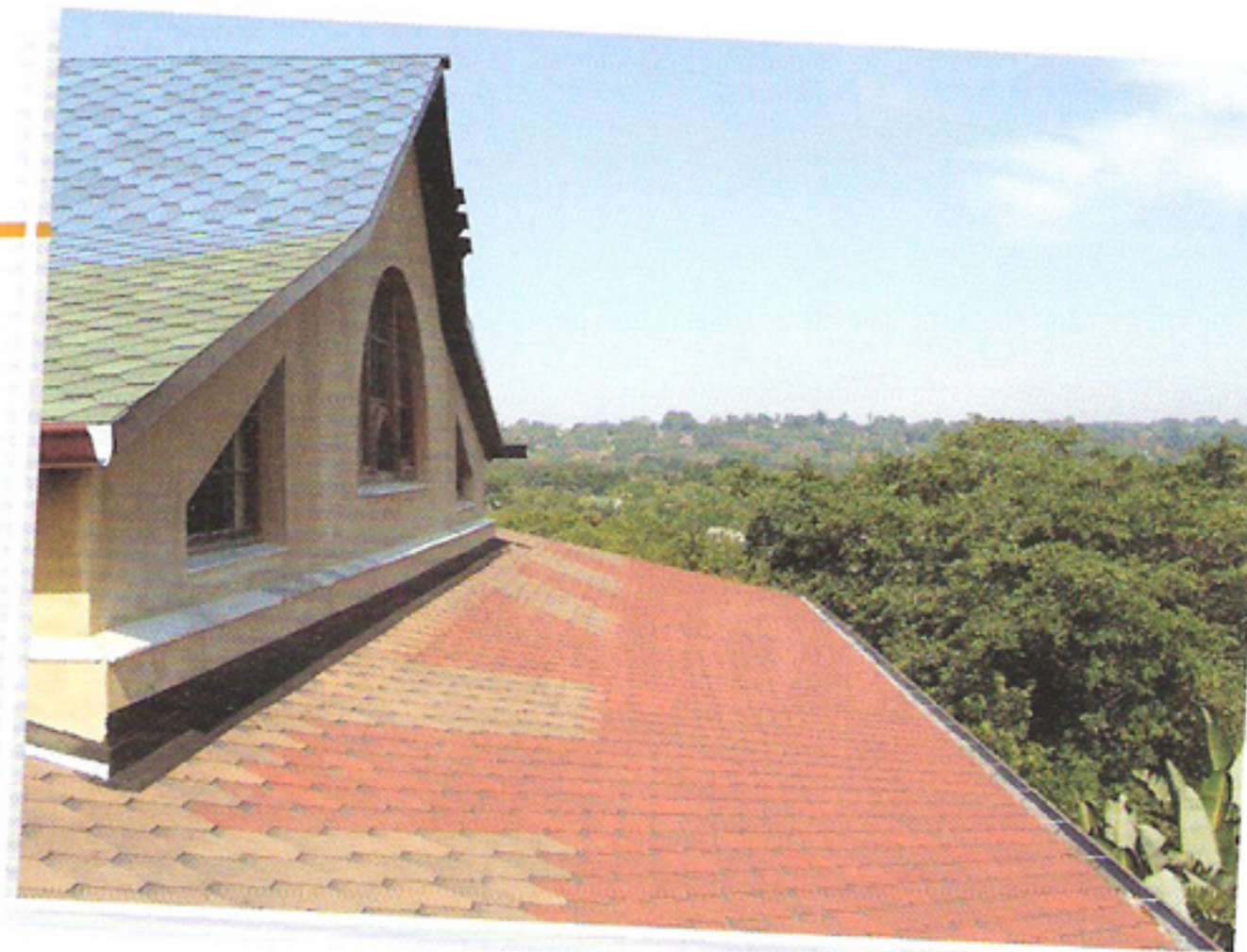
a.b.e. Construction Chemicals' Tegola Canadese roof shingles were installed in a dazzling spectrum of colours on the roof of the Amm residence in Kloof, Durban.
